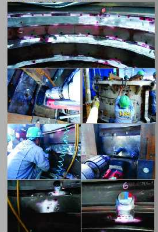
Full Torque on Turbine Casing, GTG
